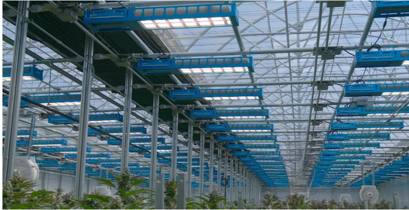
Figure 3. Pinnacle HP LED Lights in greenhouse cultivation facility
